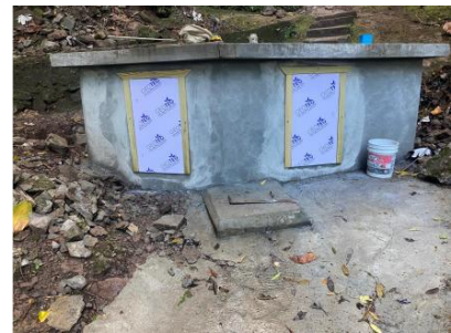
Fogarthy Springs: Larger boxes with access hatch for maintenance works.
