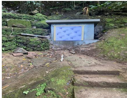
Fogarthy Springs: Stairway access leading to boxes need improvement.
