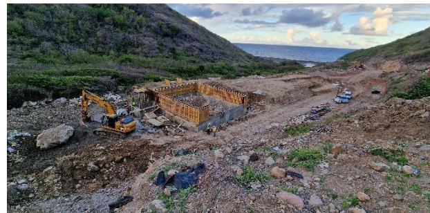
Margerita Bay Sewage Plant
